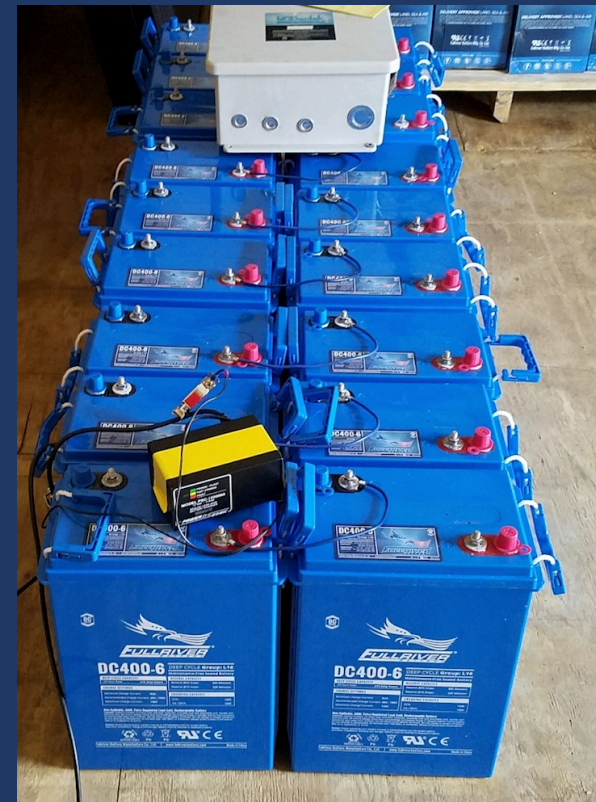
6V cells (Qty: 18) wired in series and parallel for a 12VDC system
